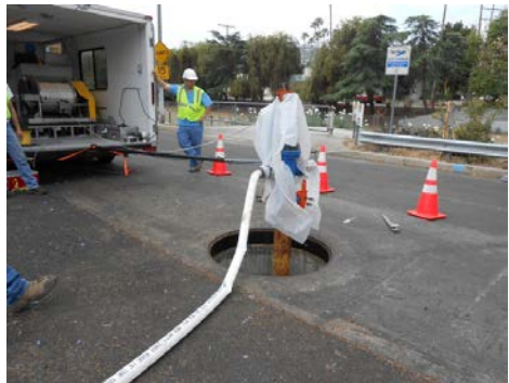
Ready to launch. The fire hose provided water to push the tool to the far end of the main. A plastic sheet contains water that leaks from the assembly. The hydrant is braced to the trailer to counteract the winching force.
