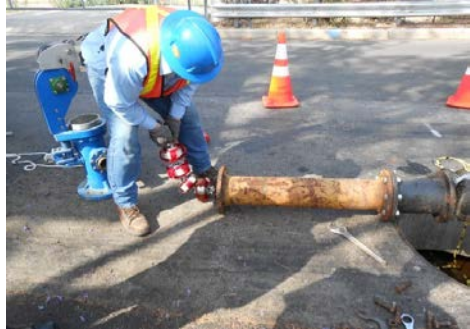
Inserting the tool into the launching port. Normally this tool is launched from a fire hydrant's vertical drop leg.
