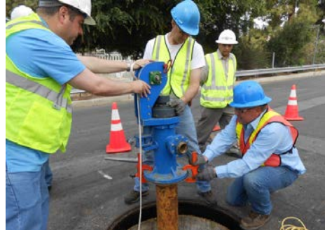
This custom hydrant guides the rope past a seal. By using clamps to hold the hydrant in place, flange patterns don't have to match.
