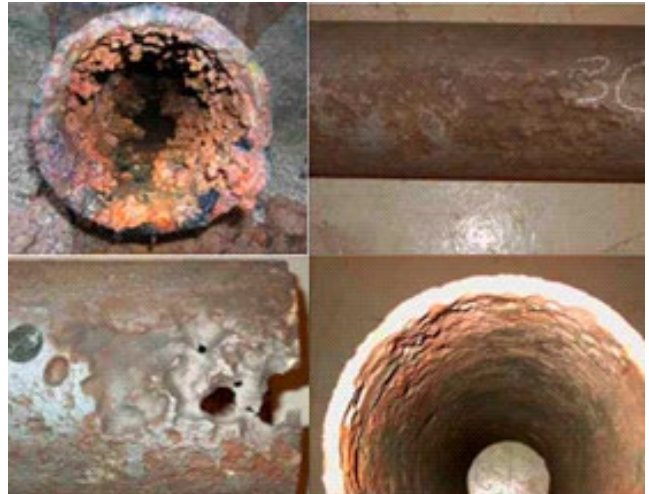
6" Cl pipe with 47% measured loss
