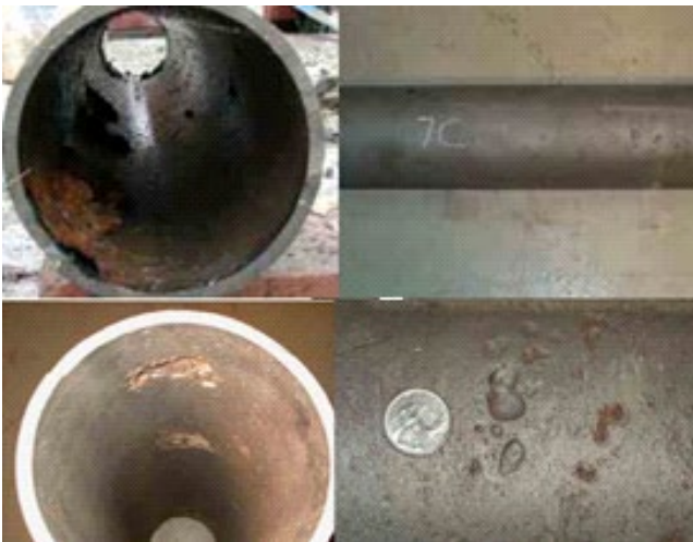
6" Cl pipe with 10% measured loss
