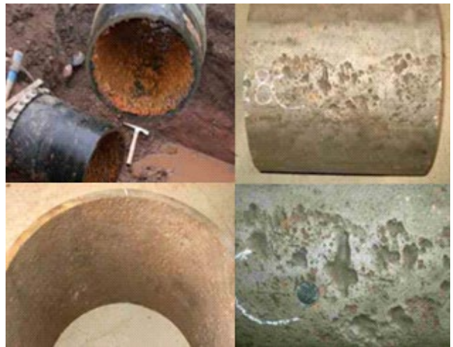
18" Cl pipe with 18.5% measured loss
