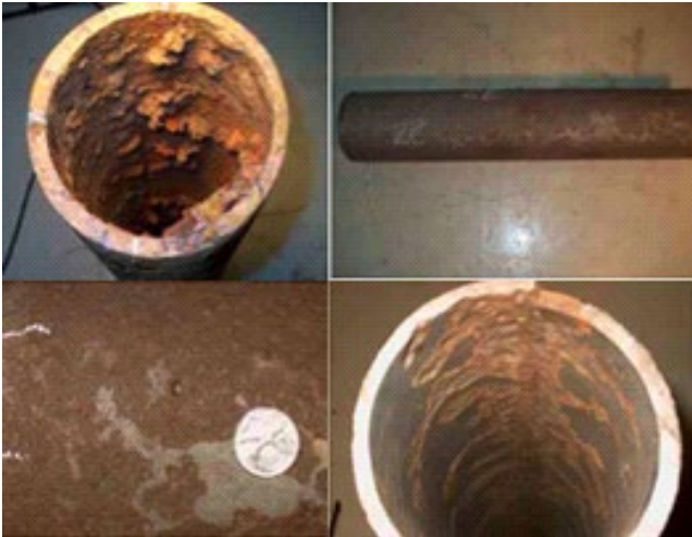
6" Cl pipe with 4.2% measured loss
