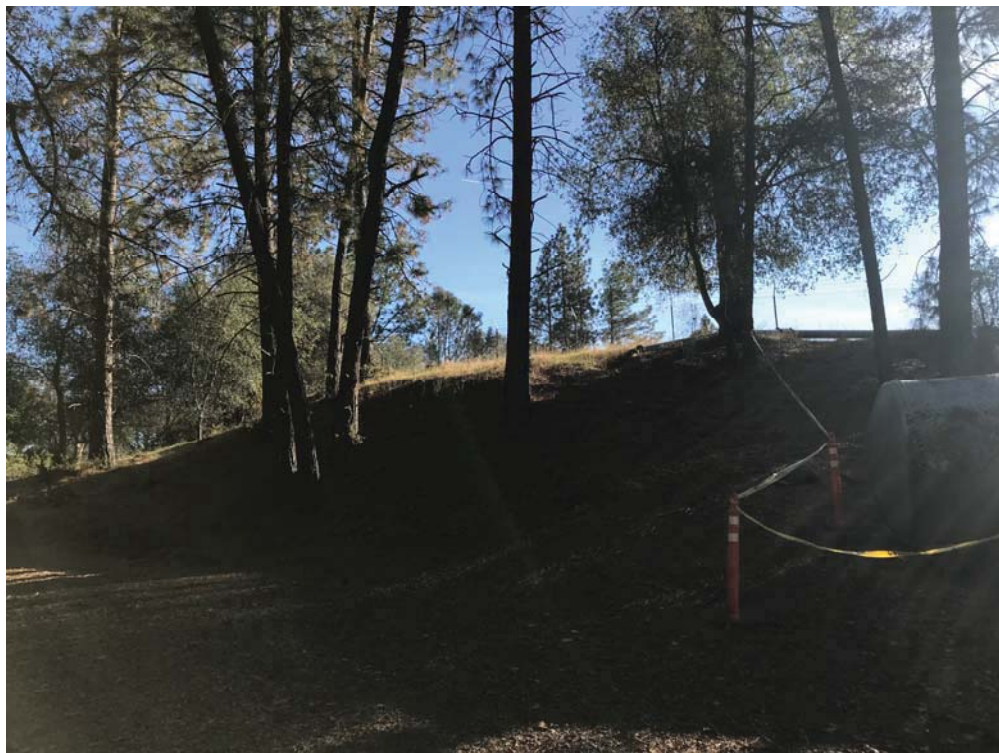
Photo #6) Slope on north side of reservoir that would be opened up as part of project construction. December 5, 2017.
